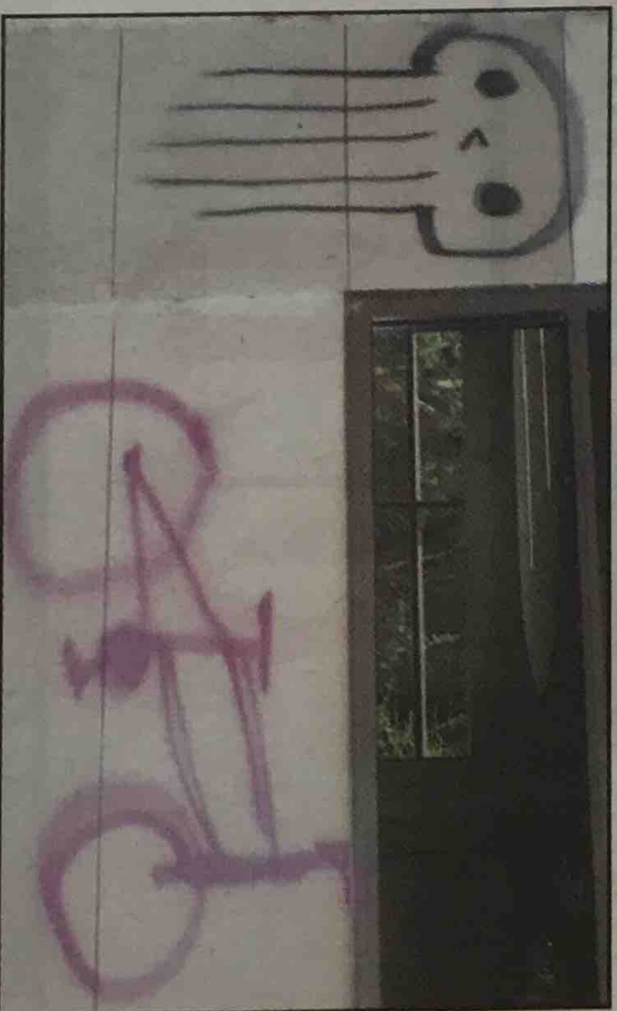
Graffiti and ob- scenities were left behind by vandals on the exterior of the new Kingwood Library. Photo by Trilla Cook
