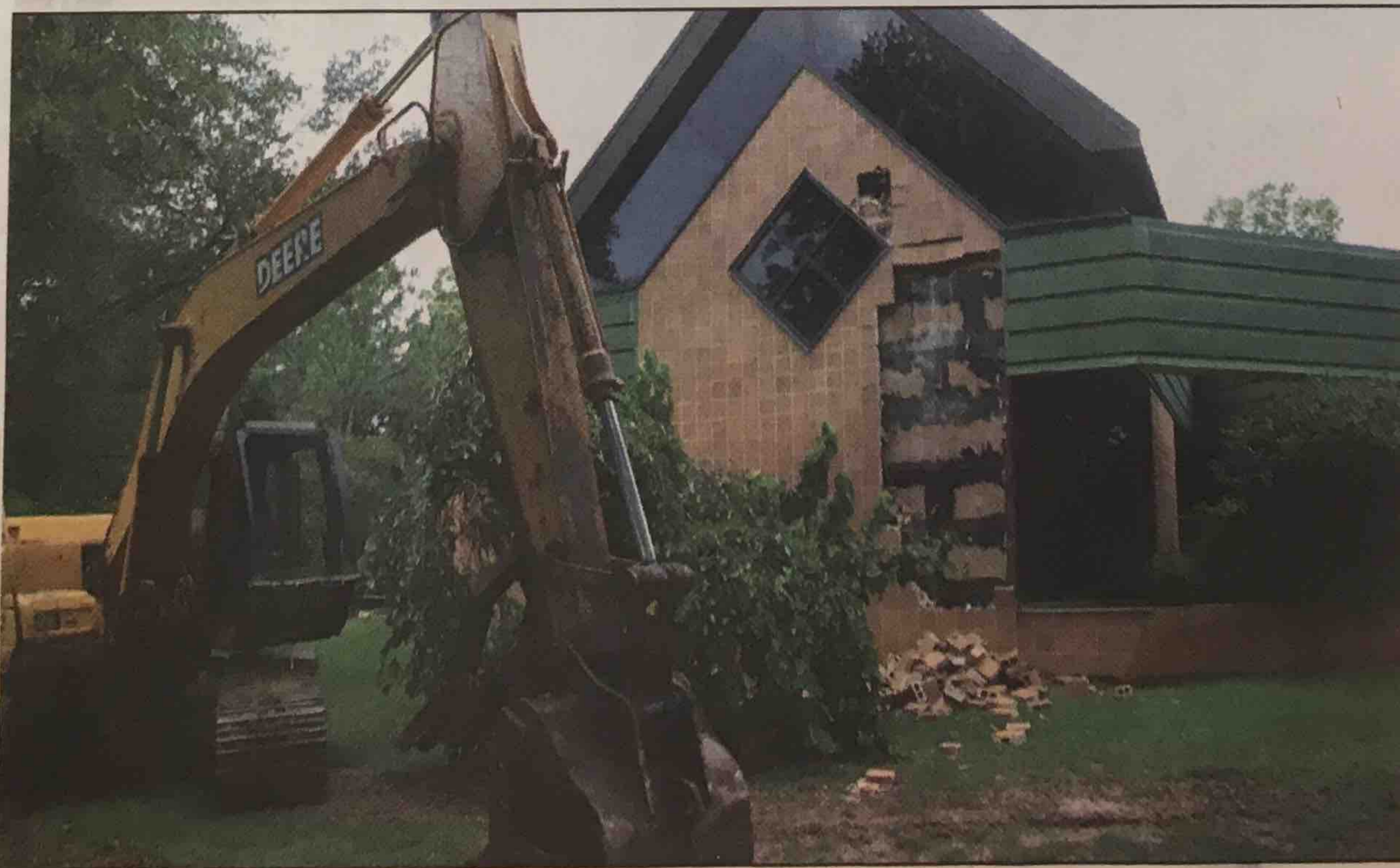
Demolition of the 'old' Kingwood library begins as crews tear down the exterior.
